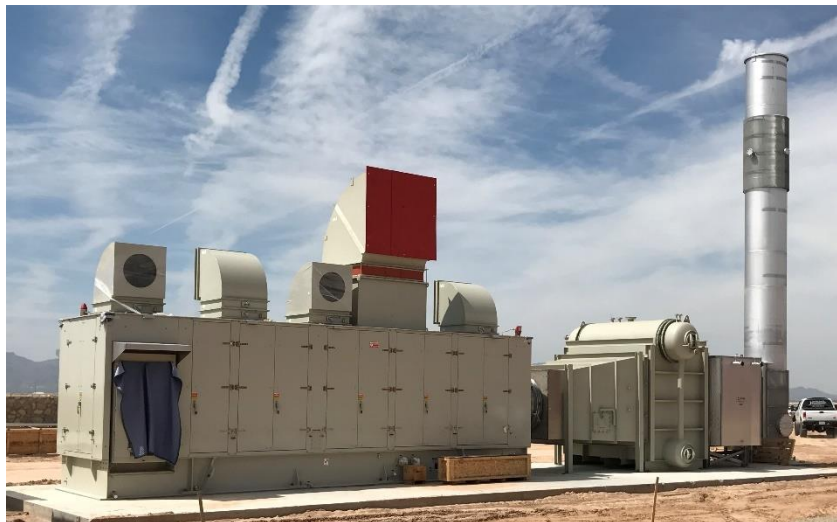
6.5 MW Natural Gas CHP
