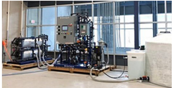
Nexed Pilot at Kay Bailey Hutchison Desalination Plant – El Paso, Texas
